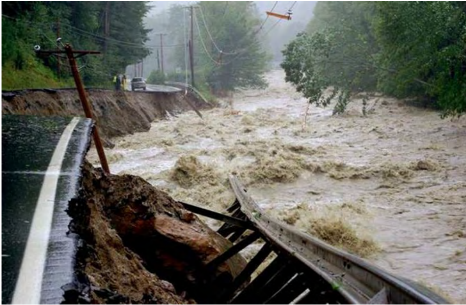
2011 Hurricane Irene (VT Route 100)
